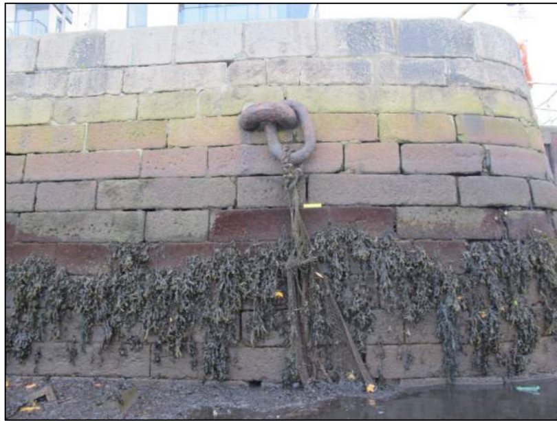
Plate 17: Oval-shaped mooring hoop inset into the quay wall at ING 318001E, 234185N (150mm scale).
