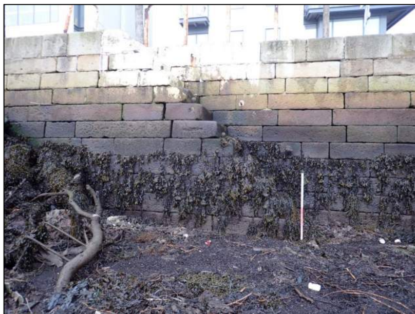
Plate 19: South-facing view of a flight of masonry river-access steps built into the north facade of the historic quay at Thorncastle Court (1m Scale).
