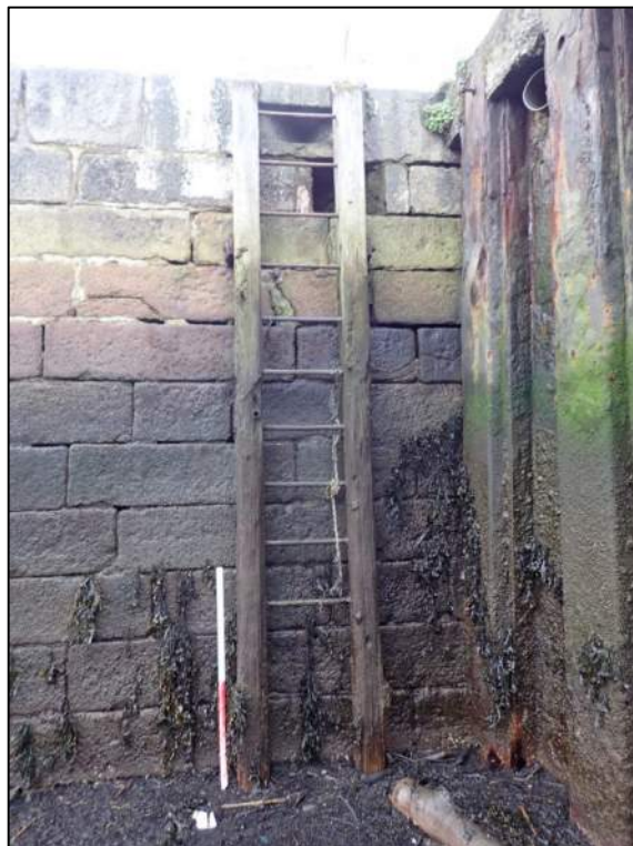
Plate 14: Timber and iron ladder that has been retro-fitted to the historic masonry quay at Thorncastle Court (1m scale).
