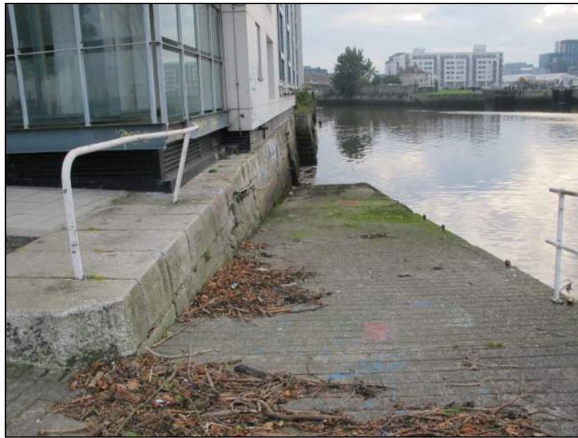
Plate 13: South-facing view of slipway (built in the 1920s) at proposed bridge landfall on the east side of the River Dodder.
