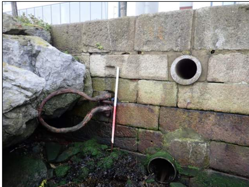
Plate 16: Southeast-facing view at interface between the masonry quays and the rock-armour that has been placed up against the structure. A large, wrought-iron, mooring hoop is positioned near the top of the quay's north facing façade at this location (1m scale).
