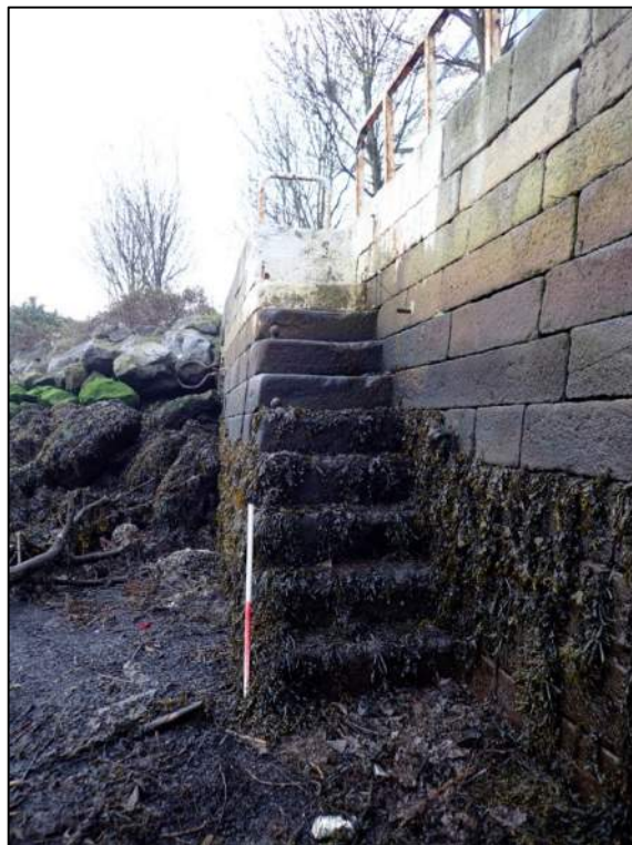
Plate 18: East-facing view of a flight of masonry river-access steps built into the north facade of the historic quay at Thorncastle Court (1m Scale).
