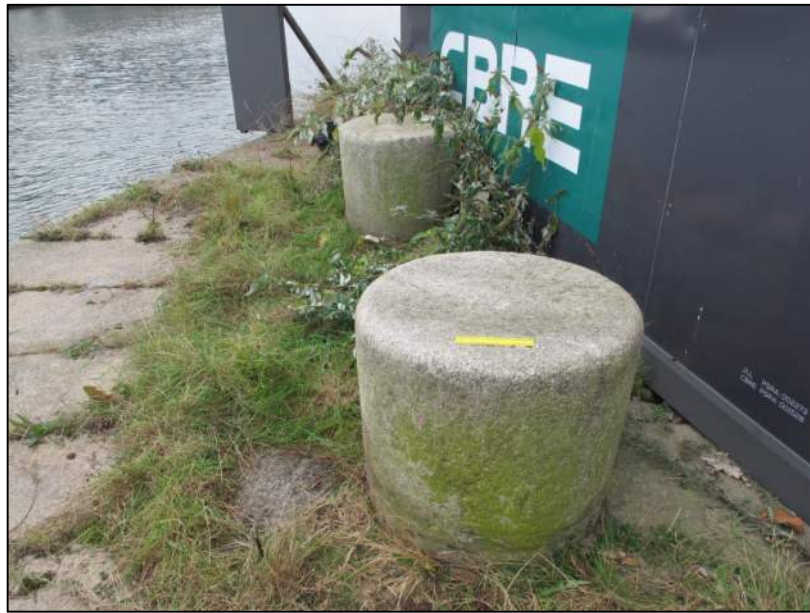
Plate 9: Pair of granite mooring-bollards inset into eastern terminus of Sir John Rogerson's Quay (150mm scale).
