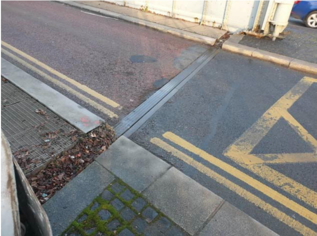
Figure 5: George's Dock Swing bridge – Expansion joint
