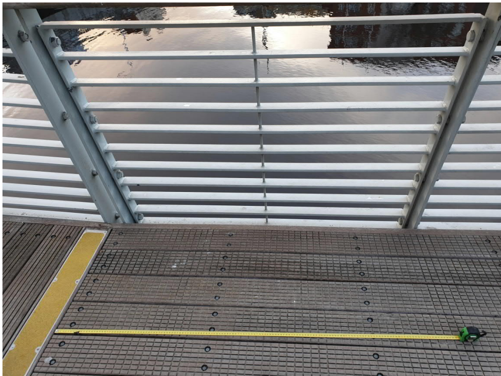
Figure 6: Cross beam spacing for the existing cantilever balcony over the River Liffey
